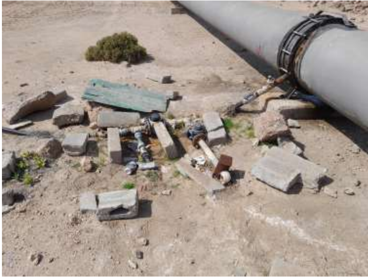
Water take-off at the Roessing pipeline
